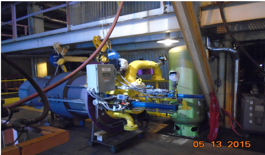
New gas burners
