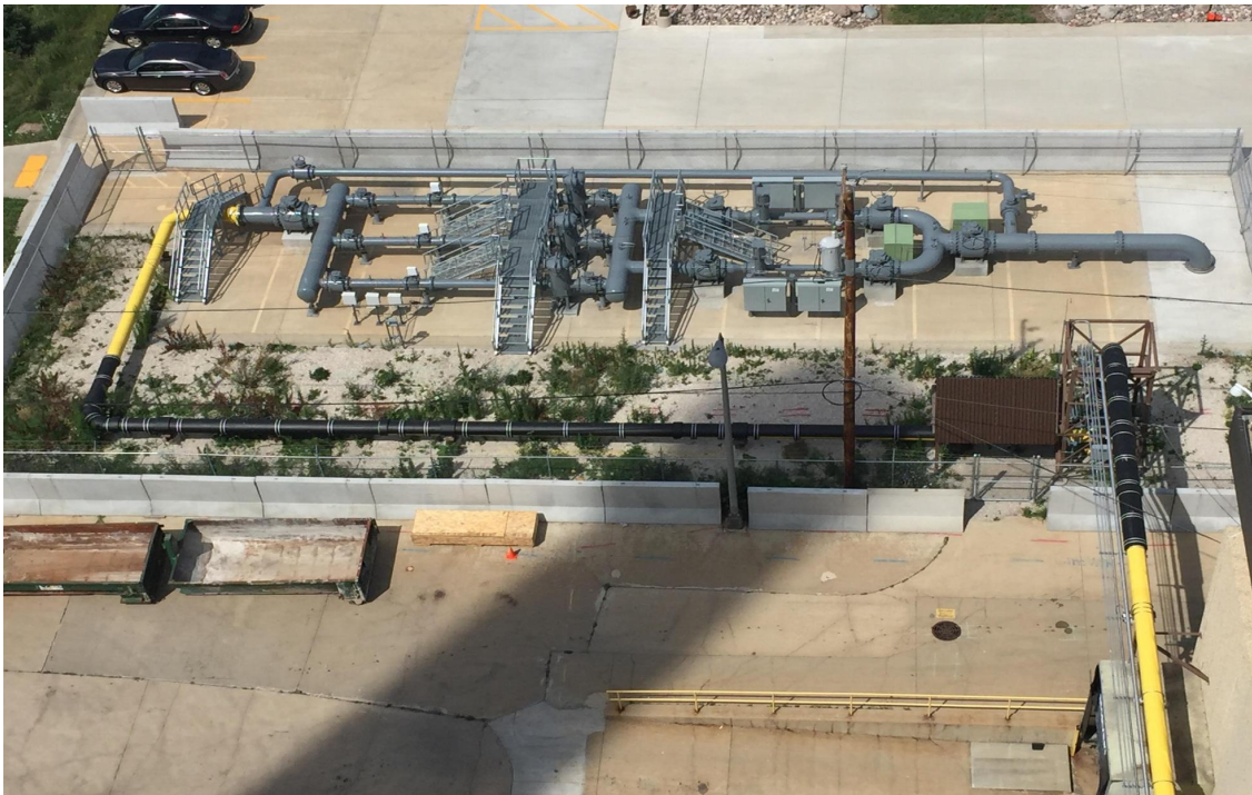
New gas regulation into the plant
