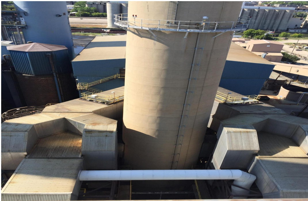
FGR ducts leading to baghouse and stack
