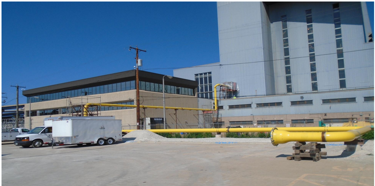
New gas lines
